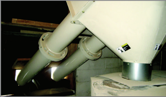
The 40 ft (12.2 m) tubular drag discharges pellets into the packaging hopper. Accumulated dust from the former rubber belt conveyor sits on top of the packaging hopper.
