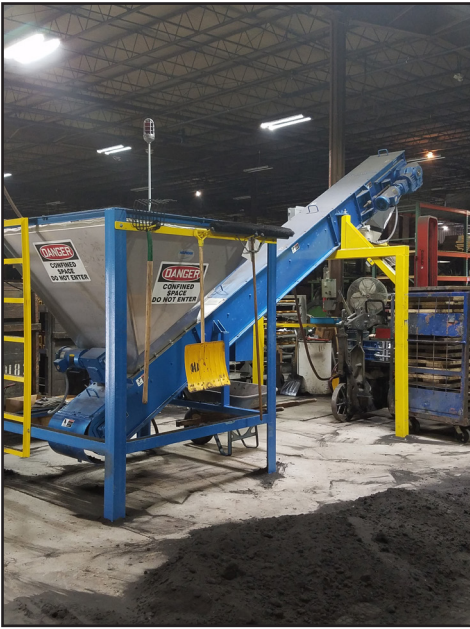
Drag Chain Conveyor engineered to efficiently and reliably move and meter the foundry sand into casting flasks.
