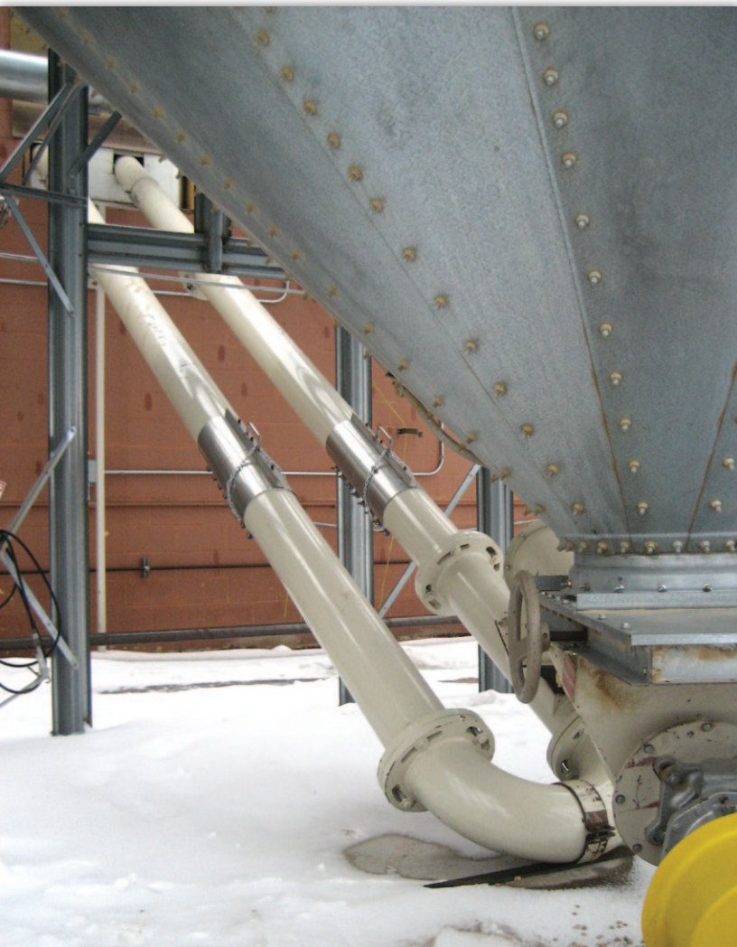
Hapman’s tubular drag conveyor reliably and gently moves 52,000 tons (47,174 metric tons) of pelletized fuel from the exterior storage silo to the interior packing line annually.
