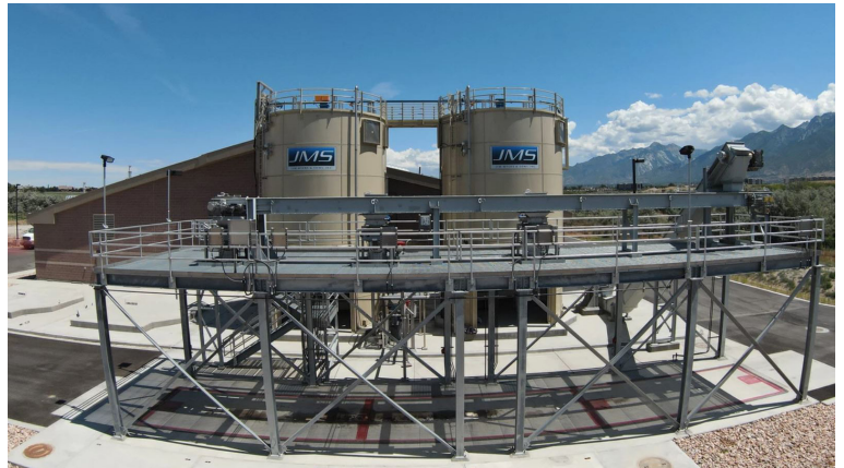
Jordan Basin Water Reclamation Facility in Utah. Two (2) Hapman Tubular Drag systems convey dried biosolids from the facility into the silo holding tanks before getting transferred via an En-Masse conveyor above a platform to be discharged into semi-trucks.
